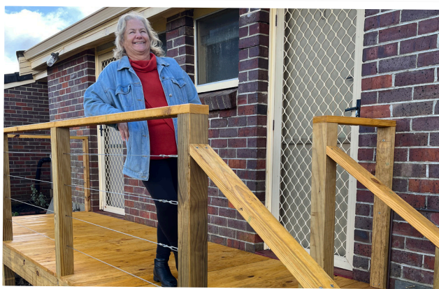
Juniper Albany Community Centre Coordinator Colleen Tombleson on a new landing and stairs making it easier and safer for residents.
